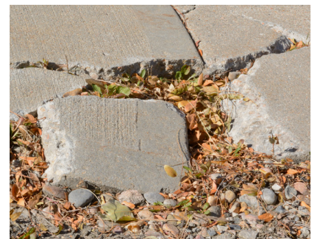
Cracked and crumbling sidewalks make walking dangerous for employees and visitors.
